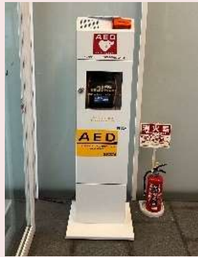
AED installation (MRR Delta Building, etc.)
